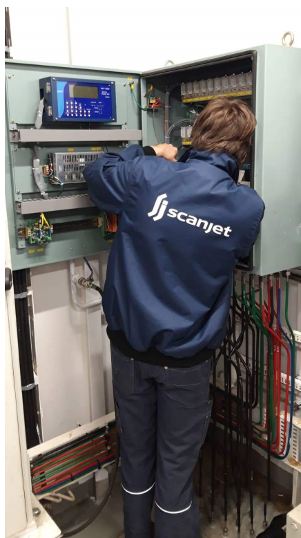
Scanjet Service Engineer installation Photo: Unknown
