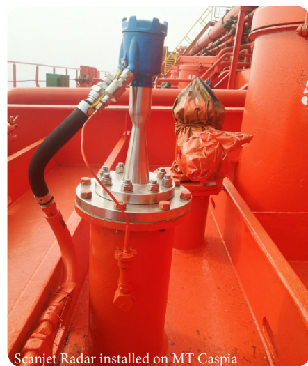
Scanjet Radar installed on MT Caspia
